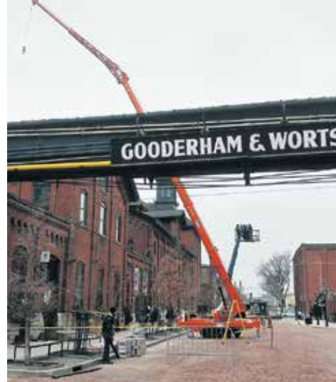
Despite its relatively small size, this Jekko SPX 1270 has a long reach. Up & Down puts the crane through its paces at the former Gooderham and Worts Distillery, now a shopping and commercial district in Toronto.
